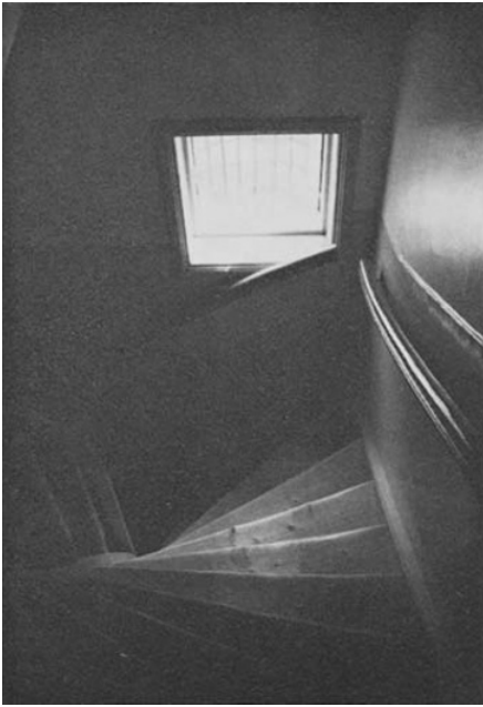
Fig. 11 FIRST BLOCK: DETAIL OF STAIR WELL FROM INTERIOR. Photograph: Dick Frank, New York.
