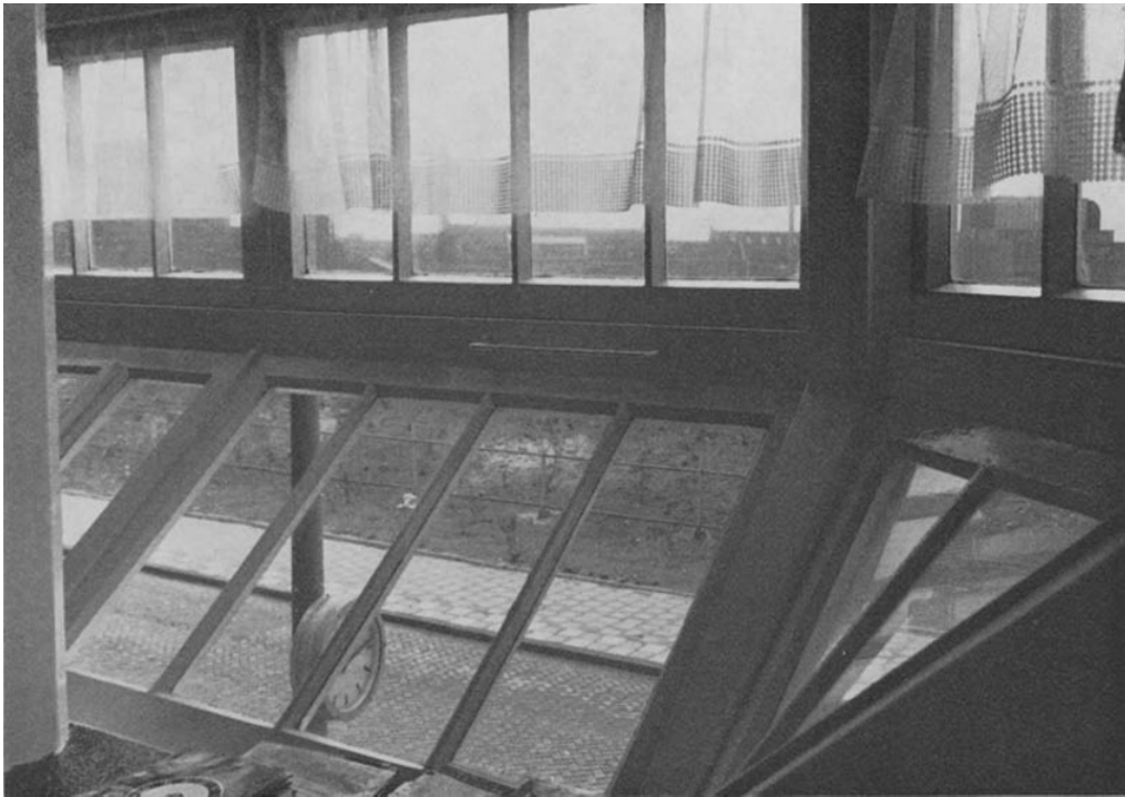
Fig. 28 THIRD BLOCK: BOWED WINDOW DETAIL: VIEW FROM INTERIOR LOOKING OUT ON ZAAANSTRAAT.
